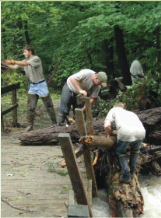
Repair of a damaged bridge at Girdled Road Reservation
